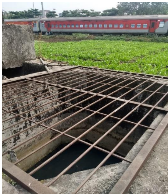
[Figure 5: Above photo depicts the dug-well constructed by the railway track farmer after the Bombay High Court banned using sewage water for irrigation.]
